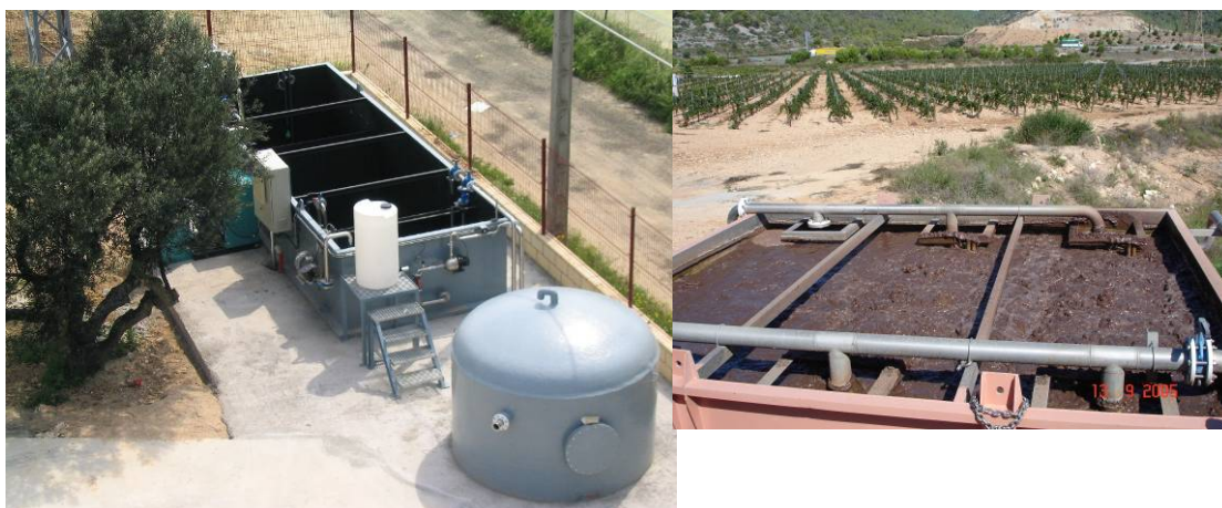
Fig. 3. Two examples of buffered compact iMBR plants in Spanish wineries.
