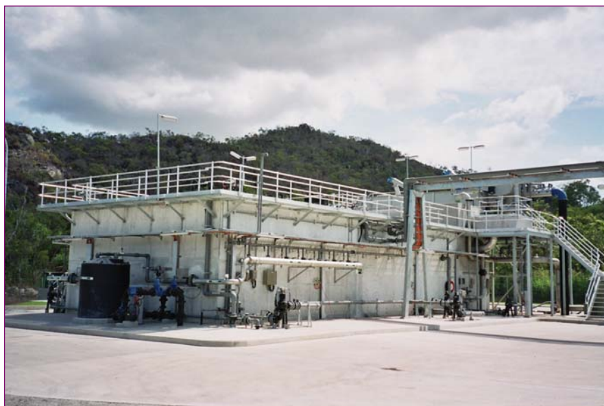
The Magnetic Island Water Reclamation (MIWR) Plant.
