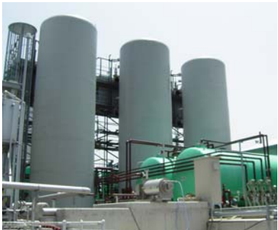
S-Company Feedstock: Alcohol stillage 60t/d Recovery of energy: Boiler
