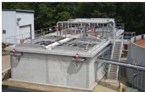
K-Company Feedstock: Salad dressing wastewater 400t/d Recovery of energy: Boiler
