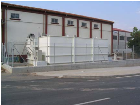
Fig 1.- General view of the plant
