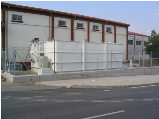
Fig 1.- General view of the plant
