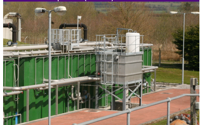
Plant Flow Splitter (below).
