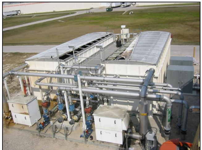
Top-view of the ADI-MBR system: 2 Membrane Tanks with Kubota ES150 units
