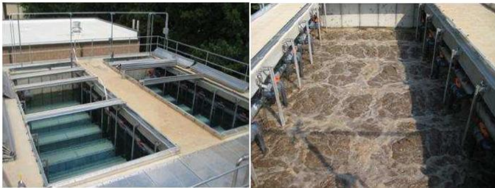
Photo of Kubota membrane units before start-up (left) and in operation (right)
